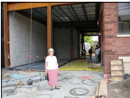
Future classrooms ( above left ), Special Education resource rooms ( above ), and new main entrance ( left ) on Hunter Avenue. WELCOME !
